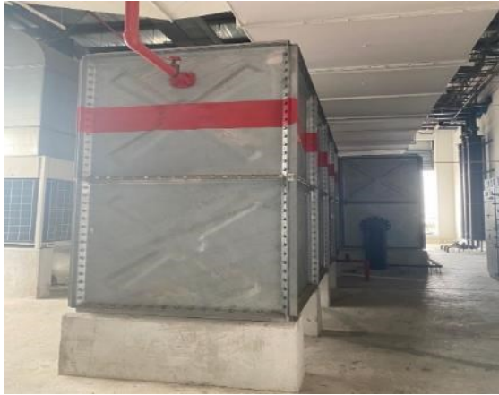
58m 3 Rainwater harvesting tank at Mi Equipment Malaysia
