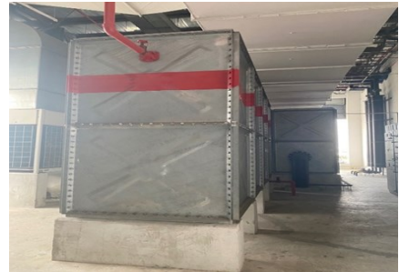
58m 3 Rainwater harvesting tank at Mi Equipment Malaysia
