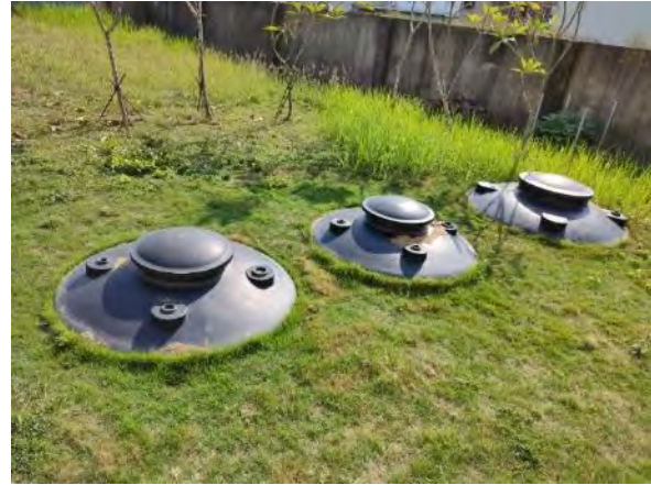
6m 3 Rainwater harvesting tank at Accurus Scientific Taiwan
